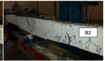
Fig. (12): Crack Pattern for B2
